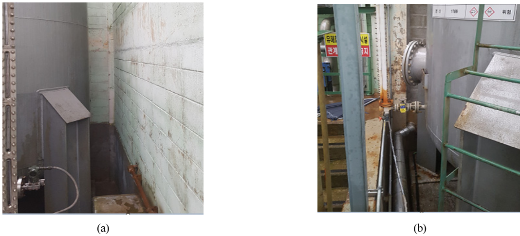
Figure 6. Facility subject to safety evaluation for noncompliance with legal requirement.
