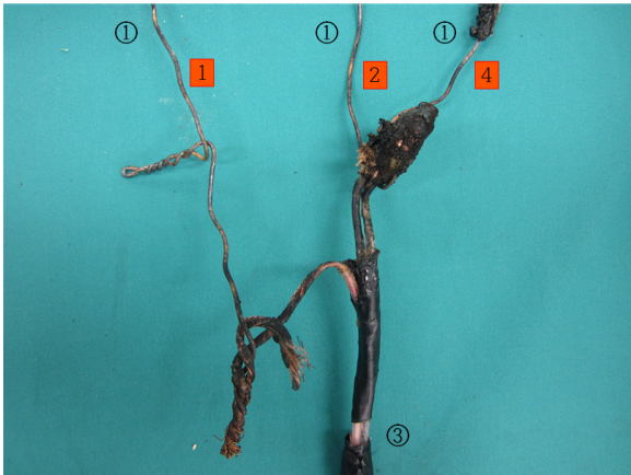
Figure 11. The Connection of ①, ②, ④ wires of ① cable and ③ cable.
