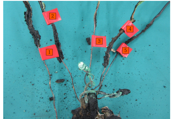
Figure 7. 5 wires of ① cable that remove carbonated coverings.
