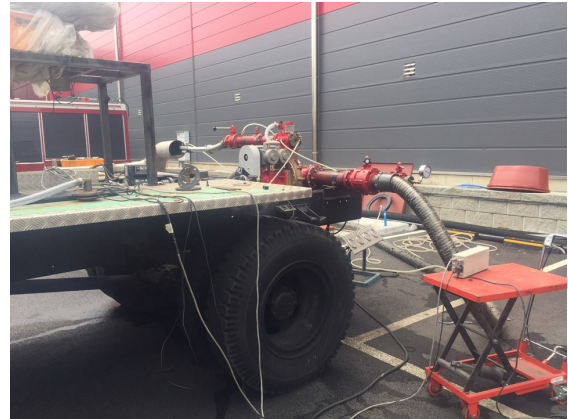
Figure 2. Current fire pump performance test on site.
